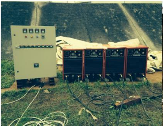
Turret 400 amp Ador Welding Machines & Power Control Pannel
