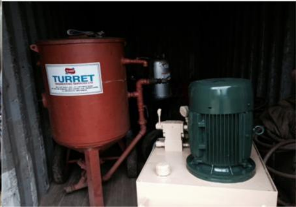
Turret Bygging Tank Jack Power Pack & Sand Pot
