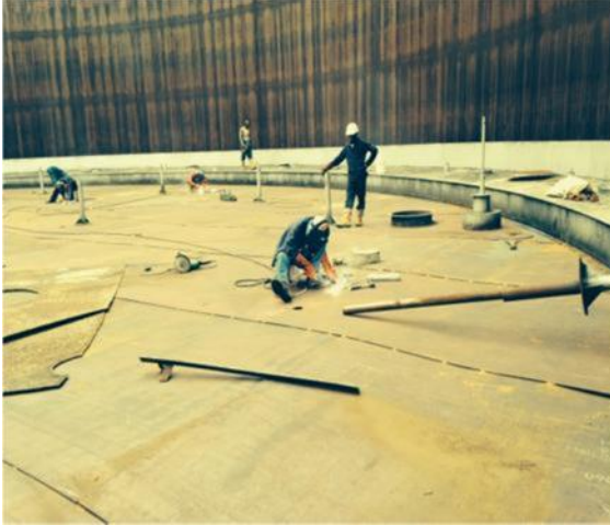
Turret Staff welding the centre deck of PHRC External Floating roof Tank 52-TK-03A
